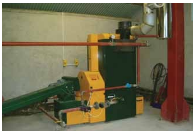
Figure 31: Integrated 120Kw KWB Boiler system (Rural Generation Ltd)
