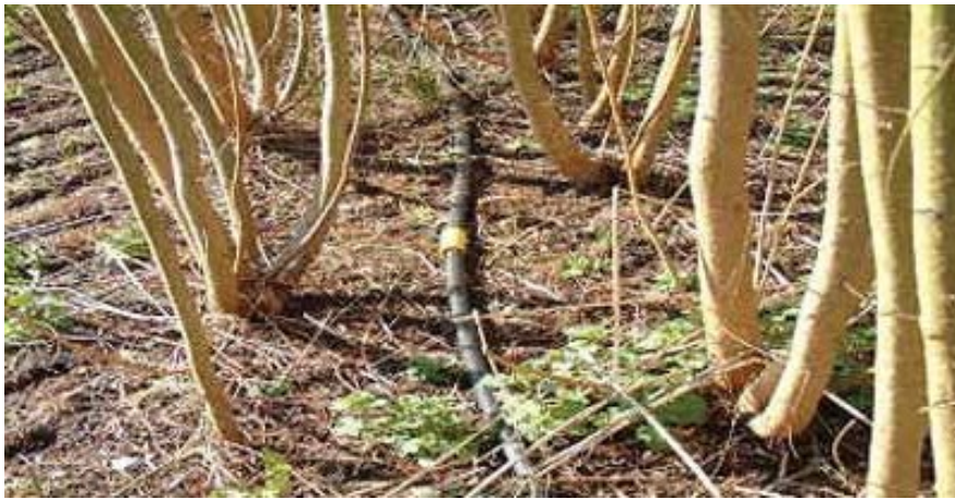
Figure 37: Installed irrigation system for bioremediation of wastewater Co. Londonderry (Rural Generation Ltd)
