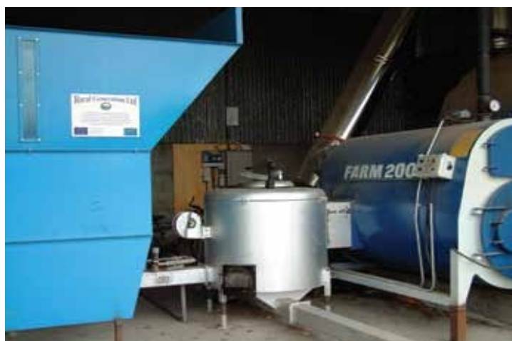
Figure 29: Swebo boiler system showing chip bunker external combustion chamber and boiler (Rural Generation Ltd)
