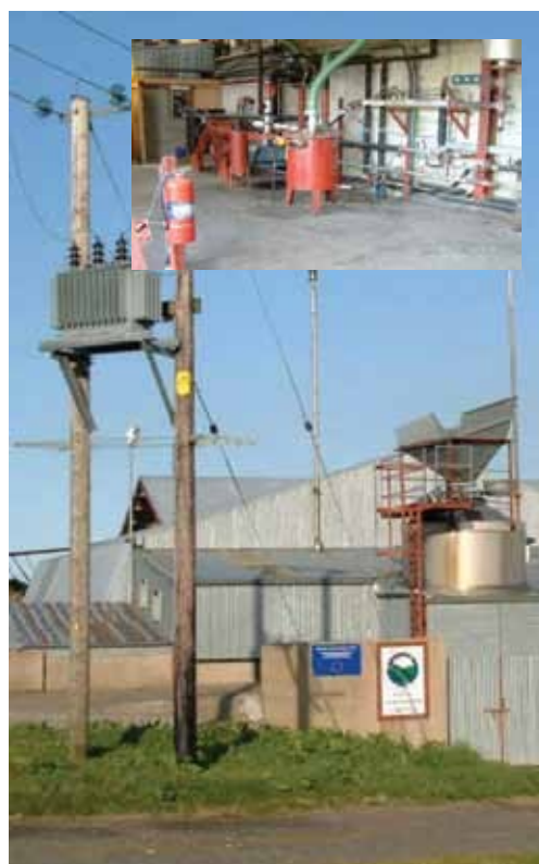
Figure 32: 100 kW Combined heat and power system using gasification (Inset showing generator and heat exchange system) (Rural Generation Ltd)
