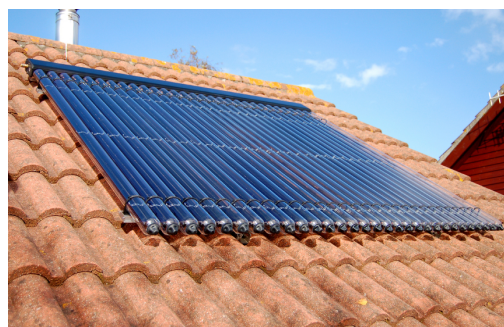
Figure 11: A typical solar hot water installation (domestic)
