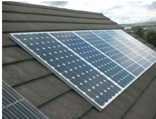
Figure 10: A typical rooftop solar PV installation (domestic)
