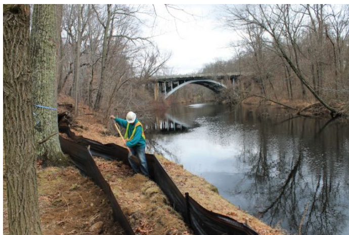
Figure 36. Silt fence installation prior to harvesting in a SMZ in Connecticut, USA (Photo courtesy of Newstimes).
