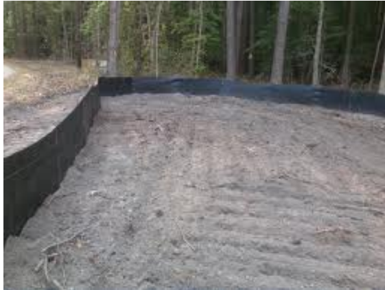
Figure 15. Water course protection measures: a) Straw wattles, b) Silt fence close-up. C) silt fence installation along a disturbed forest area. Photos courtesy of the USDA Natural Resources Conservation Service).
