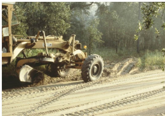
Figure 17. Constructing a road turnout, Apalachicola National Forest, Florida. (Photo by Daniel G. Neary).
