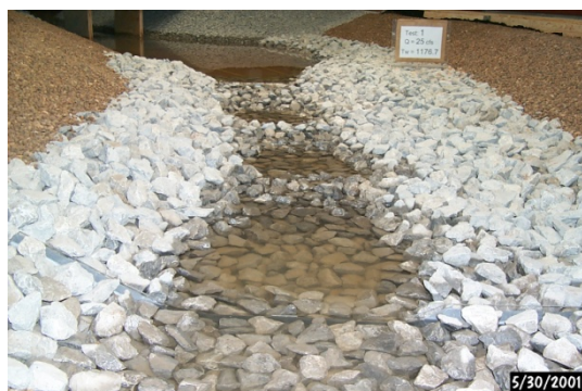
Figure 56. NRCS designed grade control structure on Sugar Creek, Franklin County, Mississippi, USA, using large rocks (Photo courtesy of USDA Agricultural Research Service).
